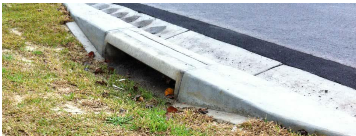
Figure 5-5 Concrete apron on grassed ZAM device avoids need for spray-strip or other edge management treatment. Source: 2018 ZAM-WSUD Handbook.
