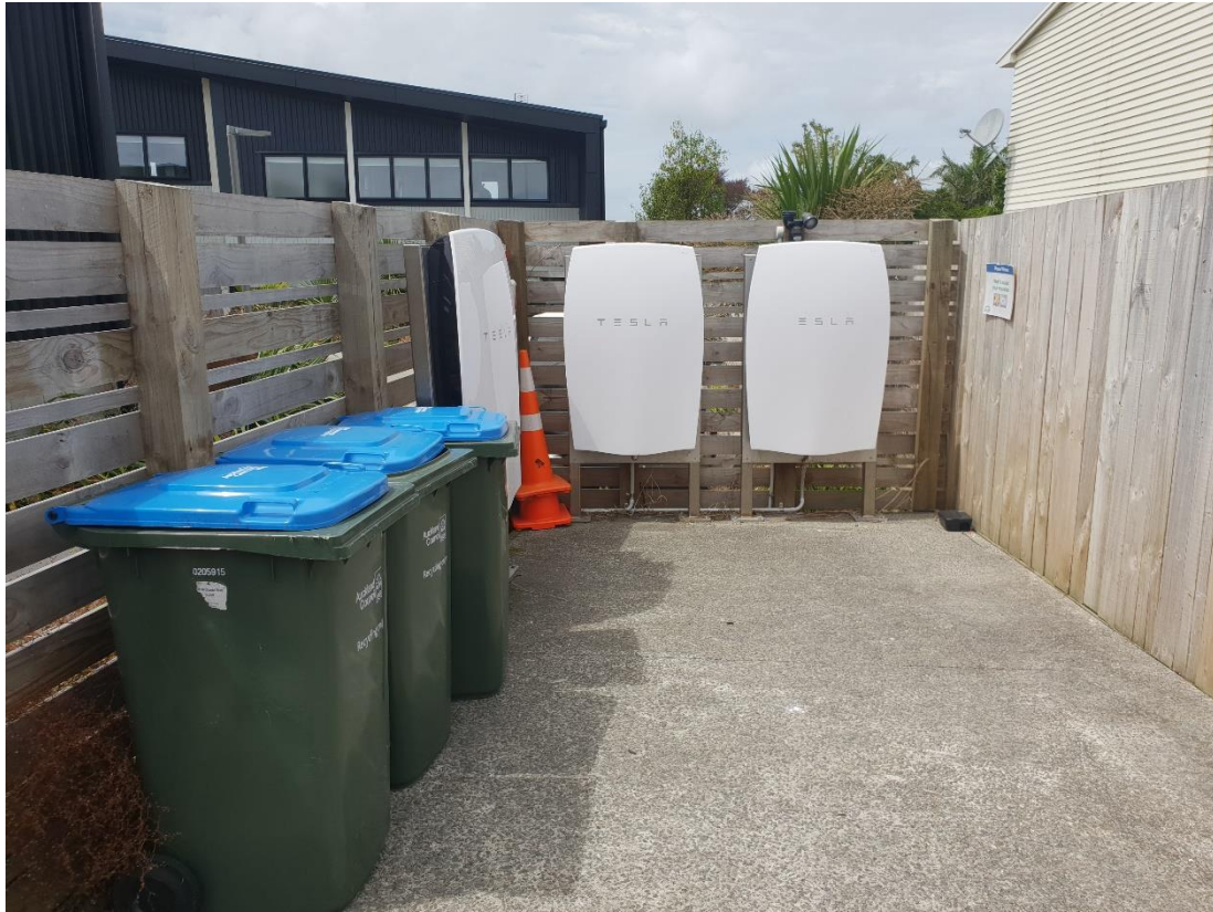
Figure 4.22: Kāinga Tuatahi (East Block) - Tesla Energy Powerwall batteries. The batteries store excess power generated from the solar panels on the rooves and return it to individual units. Some batteries are located within units themselves, while these three are located within the screened service area.
